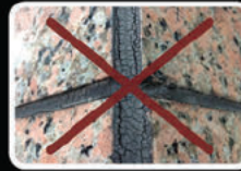
Poor UV Resistance - Sealant Cracking (PU Sealant)
