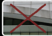
Streaking (Silicone Sealant)
